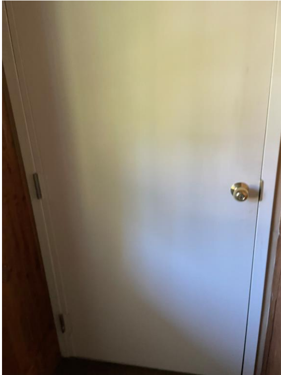
Electrical, basement door
